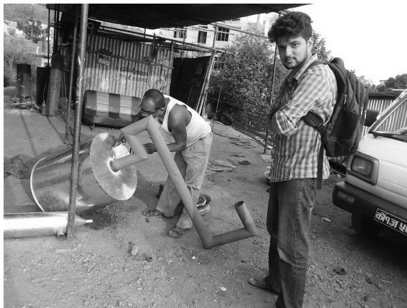
Plate 2 Welding and joining of smoke transfer pipe with settling tank
